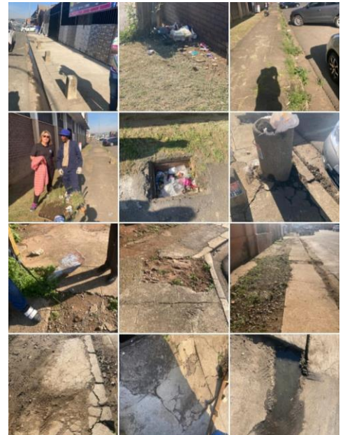
This is just one small section of Victoria Road. Besides the neglect and filth, years of zero maintenance and unrepaired excavations make it look like a war zone where bombs had exploded on the pavements..
